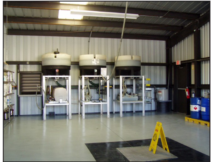
Figure 5.19: Agricultural facility with separate rinsate tanks designated for different pesticide classes. Credit: UF/IFAS Pesticide Information Office.
